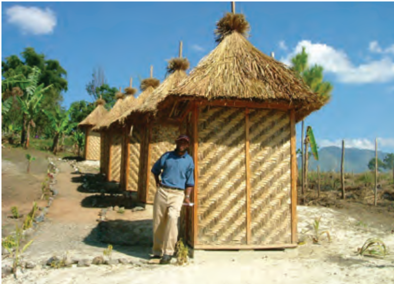
New toilets for Kintinu school in PNG, constructed with help from Oxfam
