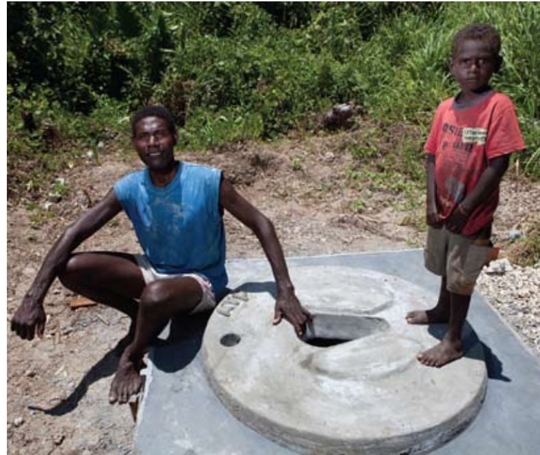
BUILDING TOILETS: Maurice Kamin and his son build a Ventilated Improved Pit latrine in Tinputz village, North Bougainville. PHOTO: TOM GREENWOOD/OXFAM
