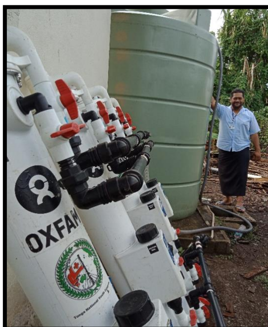
Mause Halahala of TNYC runs filtration units at a communal rainwater tank
